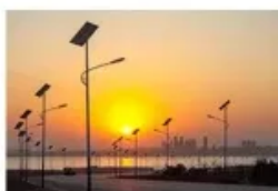
Solar Street Light
