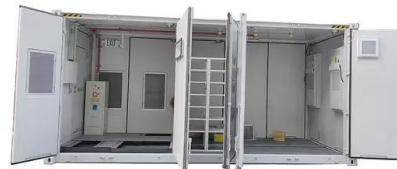
1075KW HH ESS
