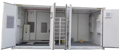
1075KW HH ESS
